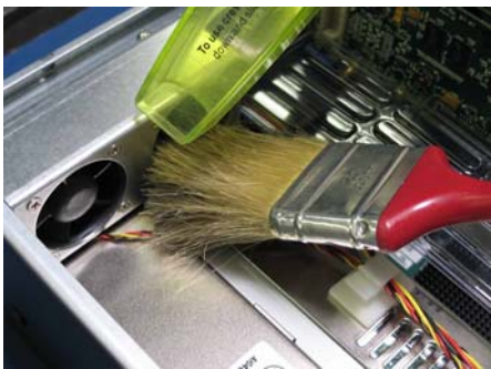
Figure 9: 1U Rear Panel Fans Cleaning
